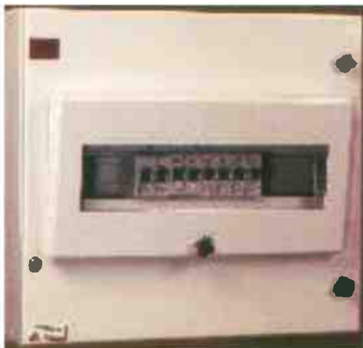
3. DC Distribution Board
